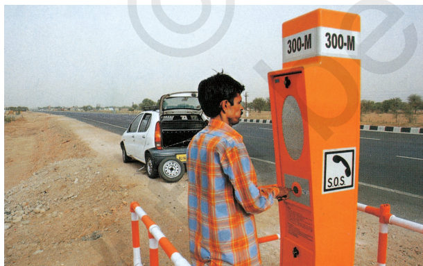
Fig.7.10 : Emergency call box on NH-8
